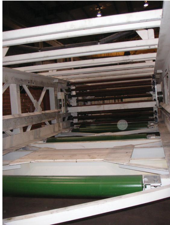
Picture 188: View into LTU unit with Return Rollers
