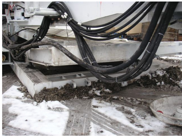
Picture 199: Floor Contact of the Mainframe
