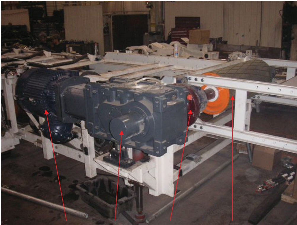
Drive Motor Gearbox Coupling Drive Pulley
