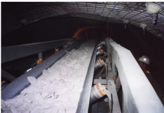
Picture 25: Underground Belt Conveyor
