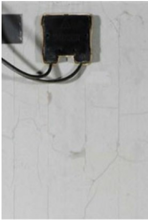
Figure 32: Module with cracking of the outer polyester layer [102]
