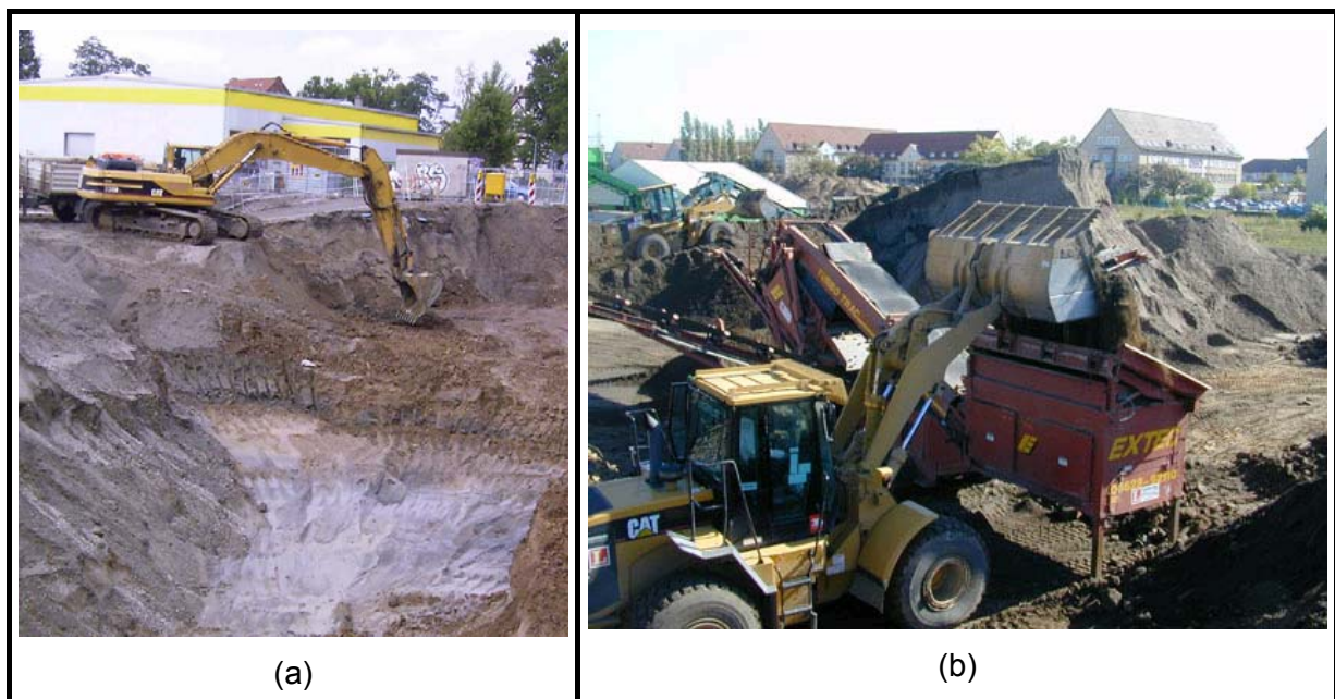
Figure 27. Phases of soil excavation: (a) Soil excavation with backhoe, and (b) Loading of the sieve facility for soil fractioning [96].
