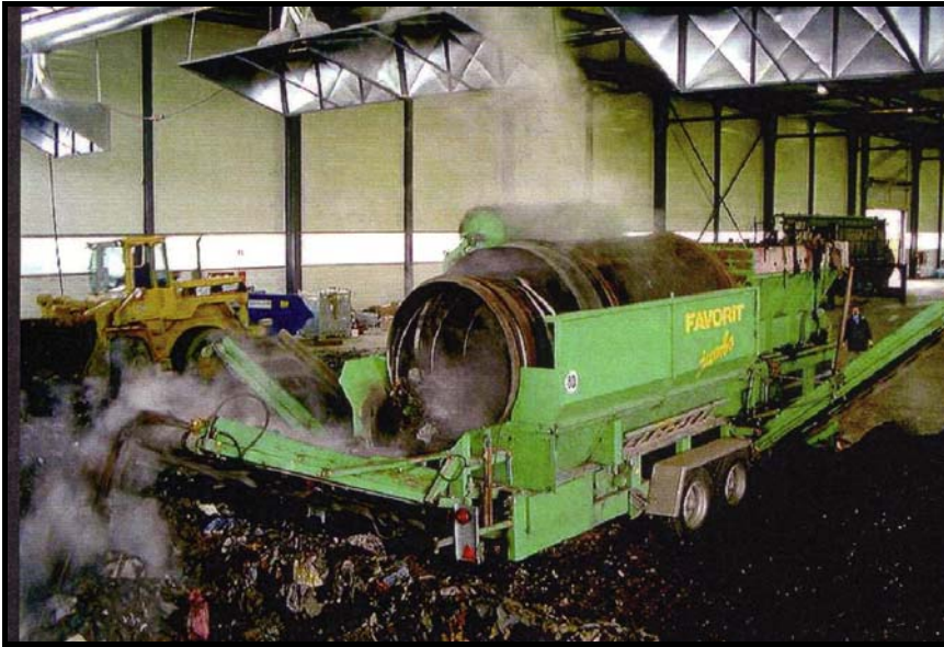
Figure 30. Drum-sieve for triage of excavated material under roof. Overview of the air extraction during the triage process.
