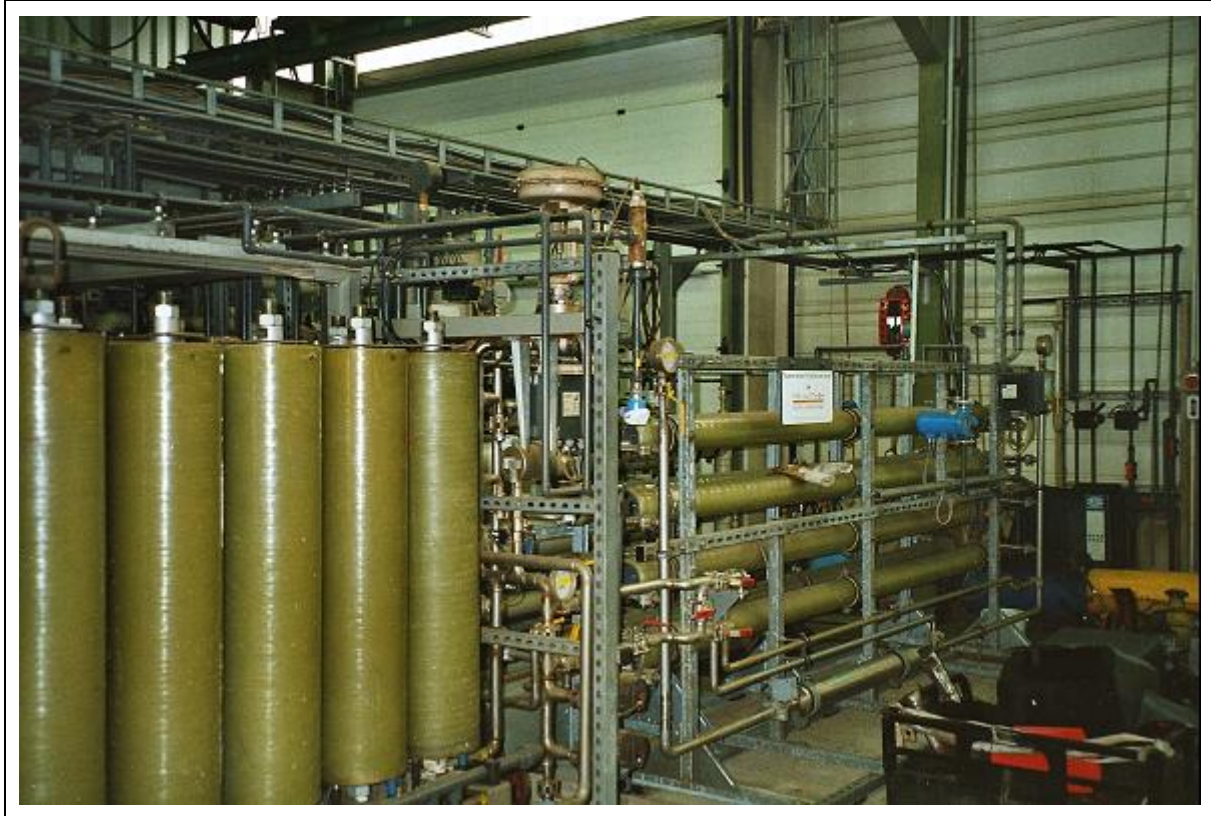
Figure VIII-6: Landfill leachate reverse osmosis treatment plant
