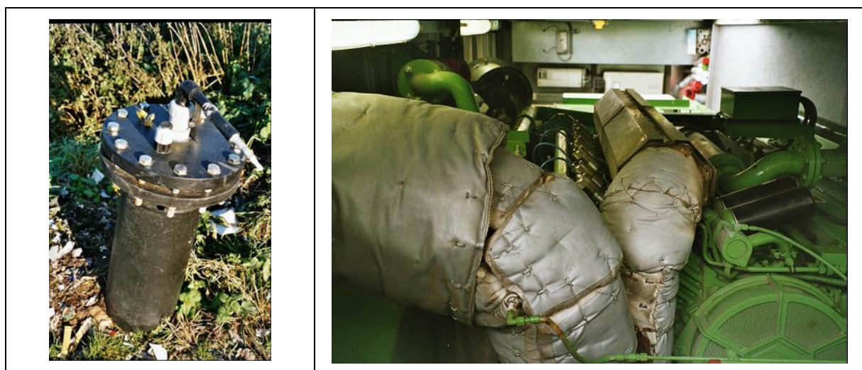
Figure VIII-5: Biogas collection and energy recovery systems
