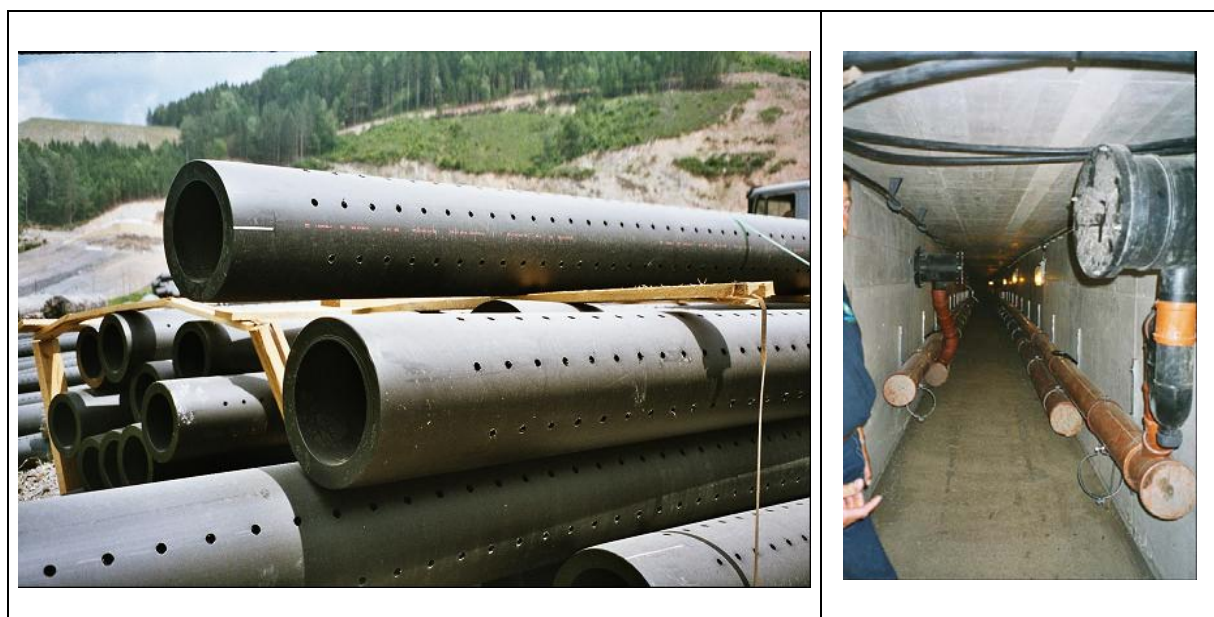
Figure VIII-4: Landfill leachate collection pipelines and pipeline configuration
