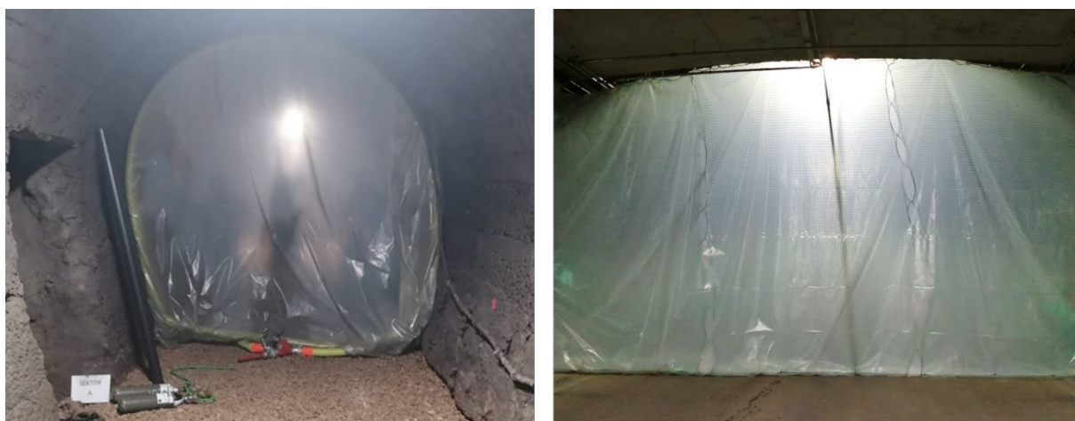
Figure 2: Left: The hose brattice - "Scheuer model" - a very easy and quick to erect option for small cross-sections (Photo: ÖBH, Scheuer). Right: Initial prototype of the mobile ventilation door made of plastic film and nets (Photo: Hofer).
